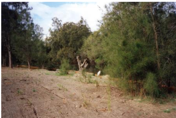
The Jones site on South Creek; jute matting laid on flood plain surface to suppress weeds, after clearance by the Green Corps, and prior to planting (NHT Grant), 2002
