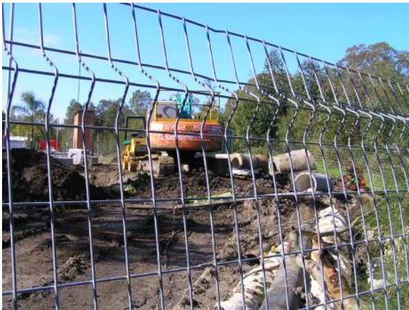
An additional sewer main was built by Hunter Water through Landcare plantings at the Jones site on the flood plain of South Creek. Funding was provided by Hunter Water for Landcare to rehabilitate the site.
