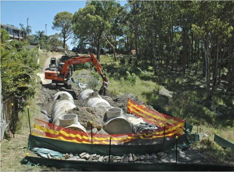
Construction of the stormwater harvesting tanks and diversion culvert. Photo from Peter Dalton.
